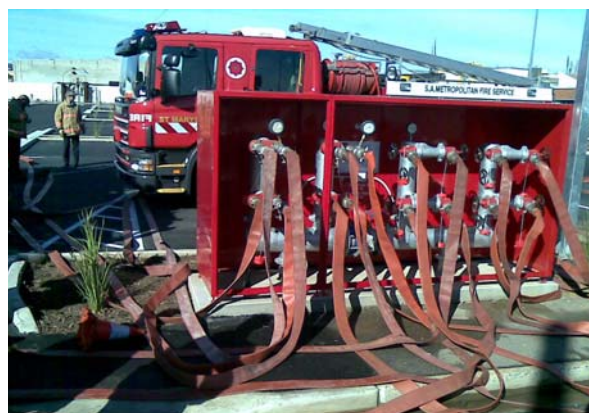
Booster testing is undertaken to ensure these systems function correctly
