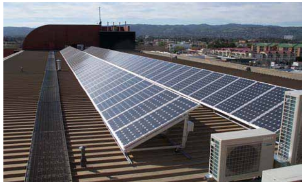
Photovoltaic cells at Adelaide Station
