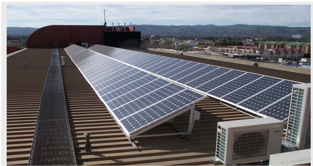
Photovoltaic cells at Adelaide Station
