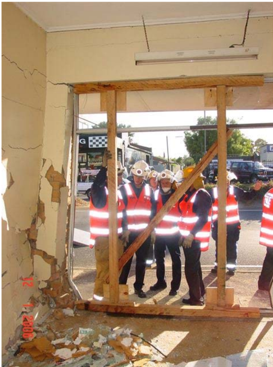
MFS officers assess the stability of a building after damage
