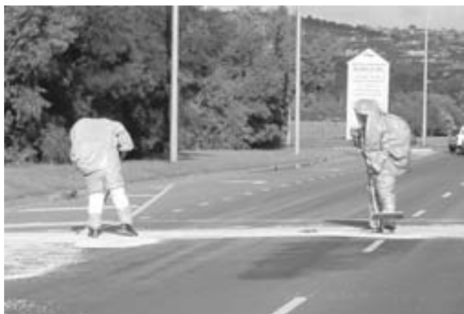
MFS Personal cleaning up a hazardous substance spillage
