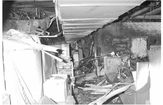
School Fire, Braeview Primary School $2.5 million deliberately lit 10 April 2004.
