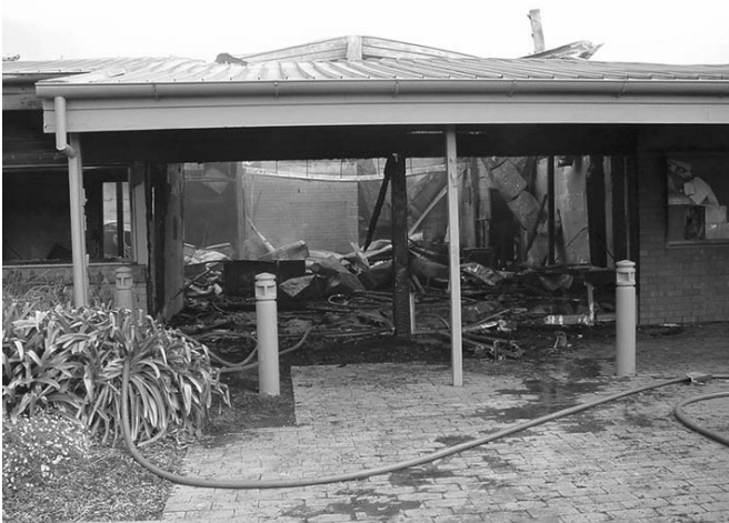
FAYS Fire, Mount Gambier The Family and Youth Services building on Elizabeth St on Thursday 22 April 2004 at 3:50 am was deliberately lit with damage in excess of $500,000. Retained firefighters took over one hour to contain the blaze.
