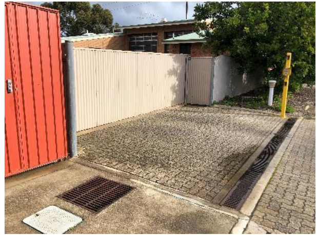
Photo 20 Drain on northern boundary of site
