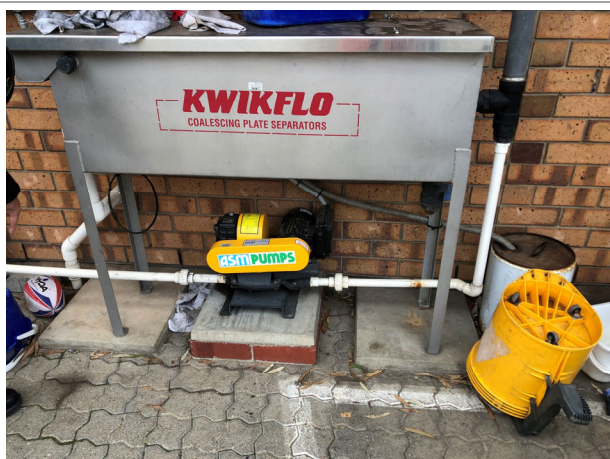
Photo 5 On site oil separator
