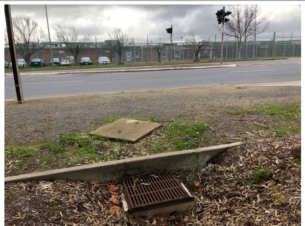
Photo 12 View of stormwater pit/ drain at site boundary on Grand Junction Road, facing north
