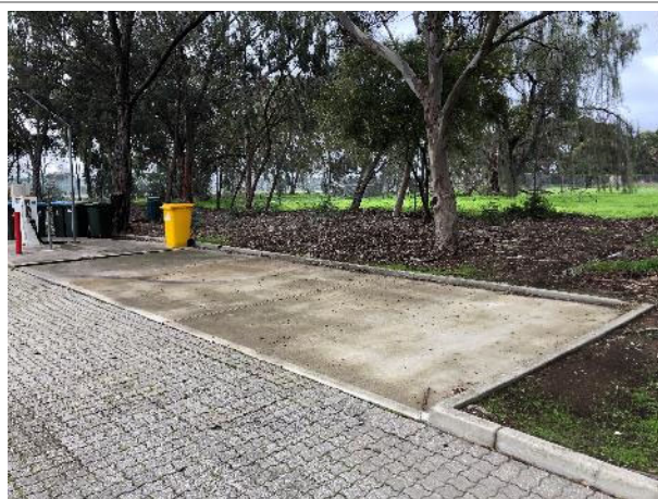
Photo 6 Former dam / fire water pump tank – backfilled and covered with concrete, facing north-east
