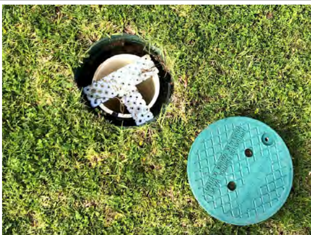
Photo 17 Groundwater monitoring well 6628-31030 – 150 mm diameter with suspended solinst data logger
