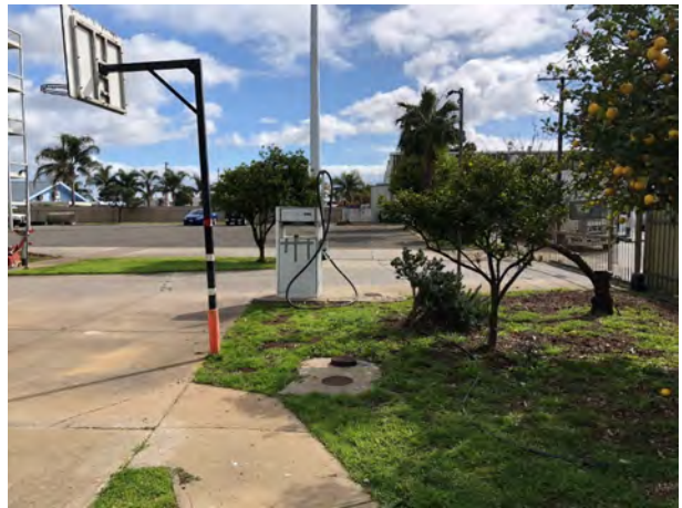
Photo 10 Diesel bowser, 8,000 L UST and fruit trees (orange, peach/nectarine and lemon) near eastern site boundary facing north
