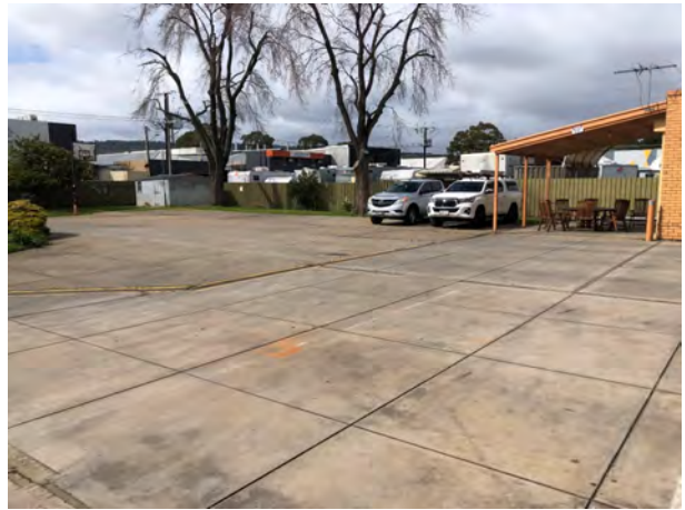
Photo 8 Rear apron / training and wash down area (concrete with cracks) off Pinn St, facing south-east
