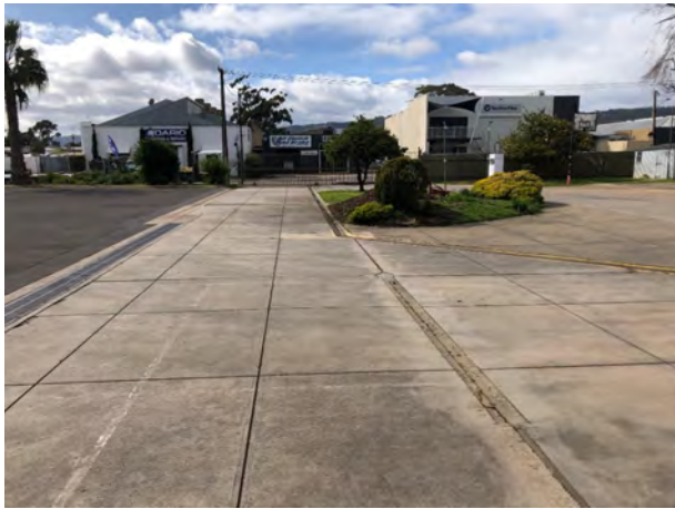
Photo 7 Rear driveway / training and wash down area (concrete with cracks) facing east towards Pinn St
