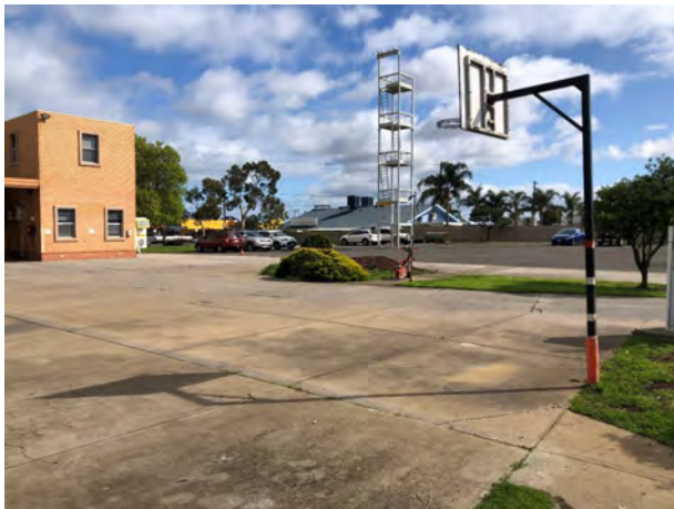
Photo 9 Training / wash down area (concrete with cracks) adjacent Pinn St in the south-eastern portion of the site, facing north-west
