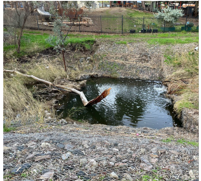
Photograph J: Christie Creek near SW12 showing rock gabions, stepped structure and some bank erosion.
