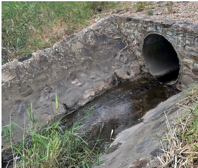
Photograph G: Another stormwater drain discharging into Christie Creek (adjacent to Photograph F), 750 m north-west of the fire station, near SW03. Potential drain where stormwater from site would discharge. Dry weather conditions.
