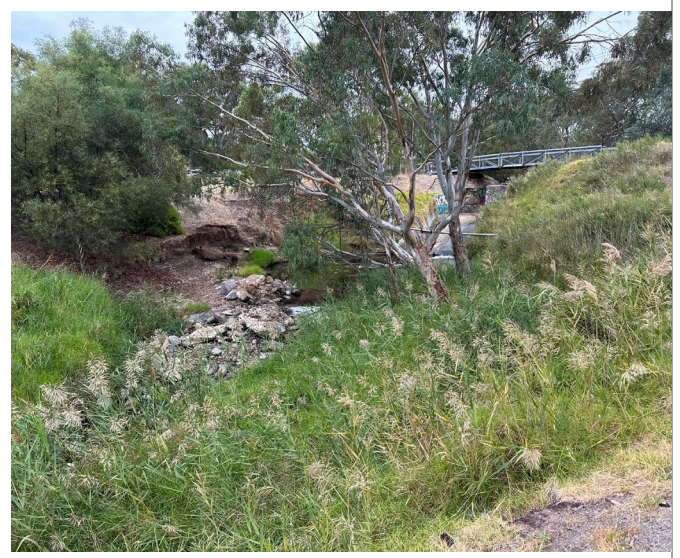
Photograph H: Christie Creek near SW01/SW11 and east of Dyson Rd, showing concrete bank and some erosion. Dry weather conditions.
